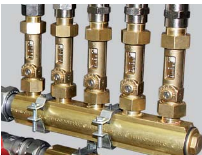
Five separate cooling circuits
